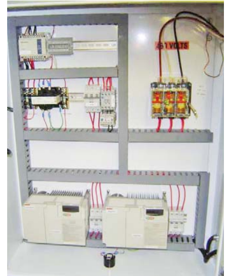
MAIN CONTROL PANEL (INSIDE)
